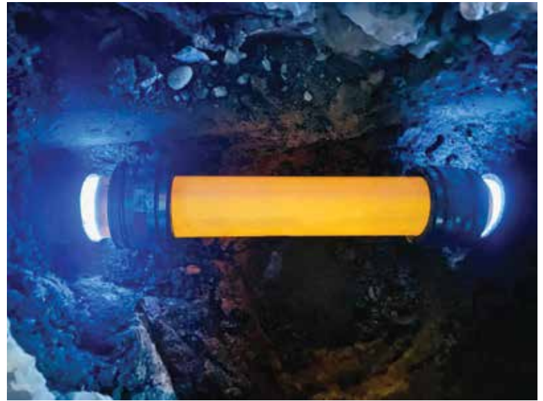
LightRay LRI was able to cast 47 feet of 4-inch pipe in 10 minutes at this job, according to Josh Shelton.
