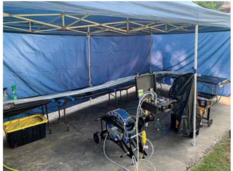
Job sites can be simplified with UV systems like the LightRay, meaning there's less equipment for crews to operate and a smaller zone to control.
