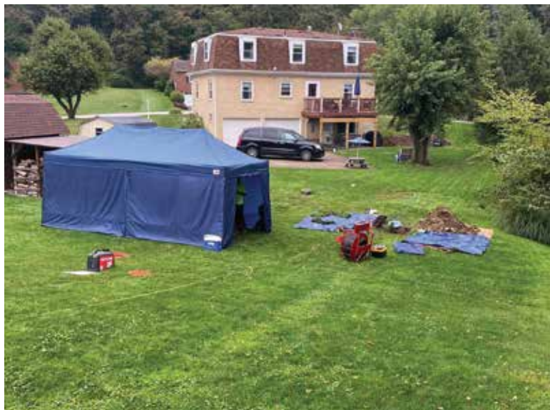
The LightRay's shorter casting time and simplified job site allow Shelton Plumbing to streamline its pipe lining process and get more jobs done in a day.
