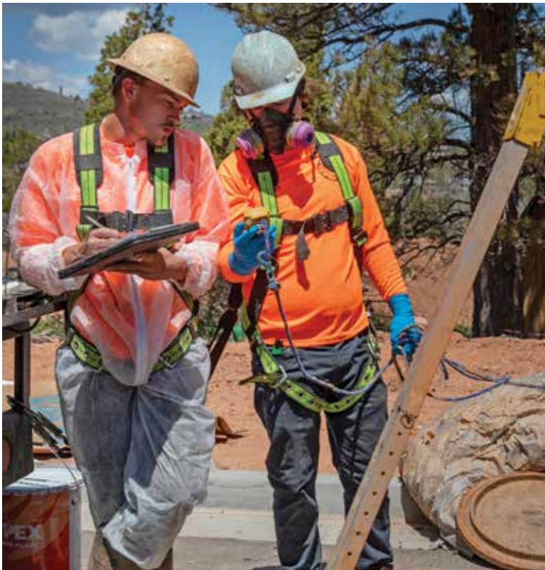
Austin Huggins (left) and Skyler Hanges record air quality data inside a new manhole using a GasAlertMax XT II detector by Honeywell Safety and Productivity Solutions.
