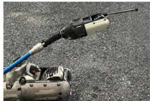
A gas line that penetrates a sewer/storm line can rupture with explosive results!
