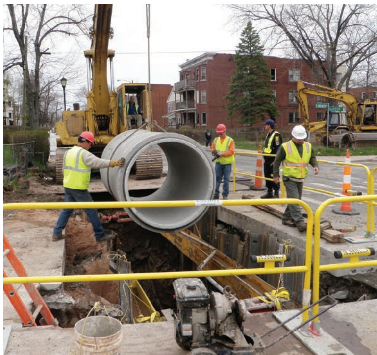
During a sewer separation project in Hartford, workers add a second pipe in the street to serve as a sanitary sewer.
