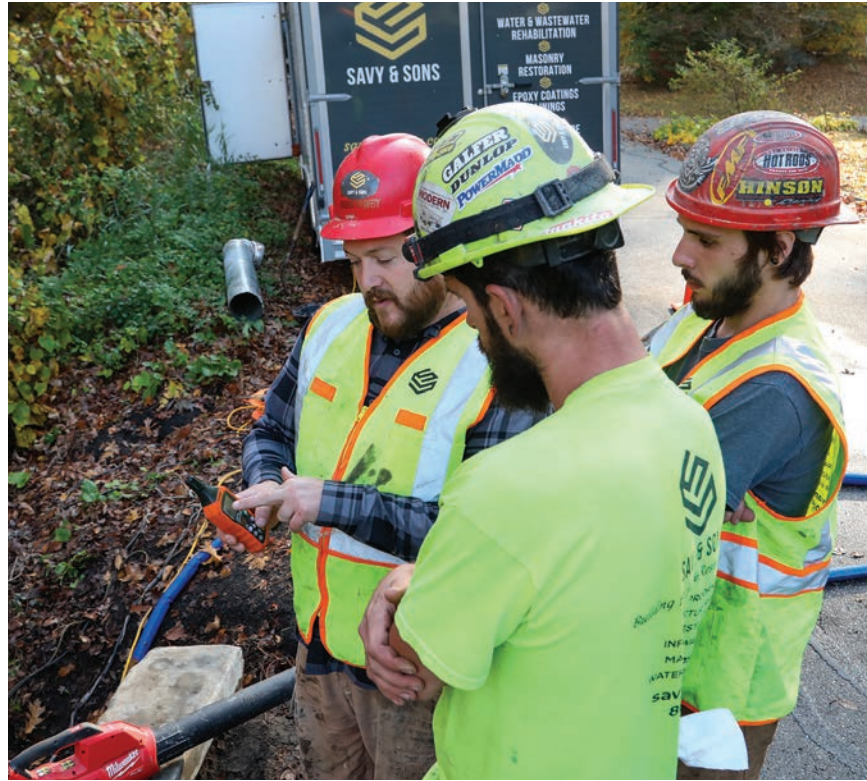
From left, Ralph Savy, Gordon Sime and Dillon Fournier discuss details of an epoxy rehabilitation of a culvert in Ledyard, Connecticut.
