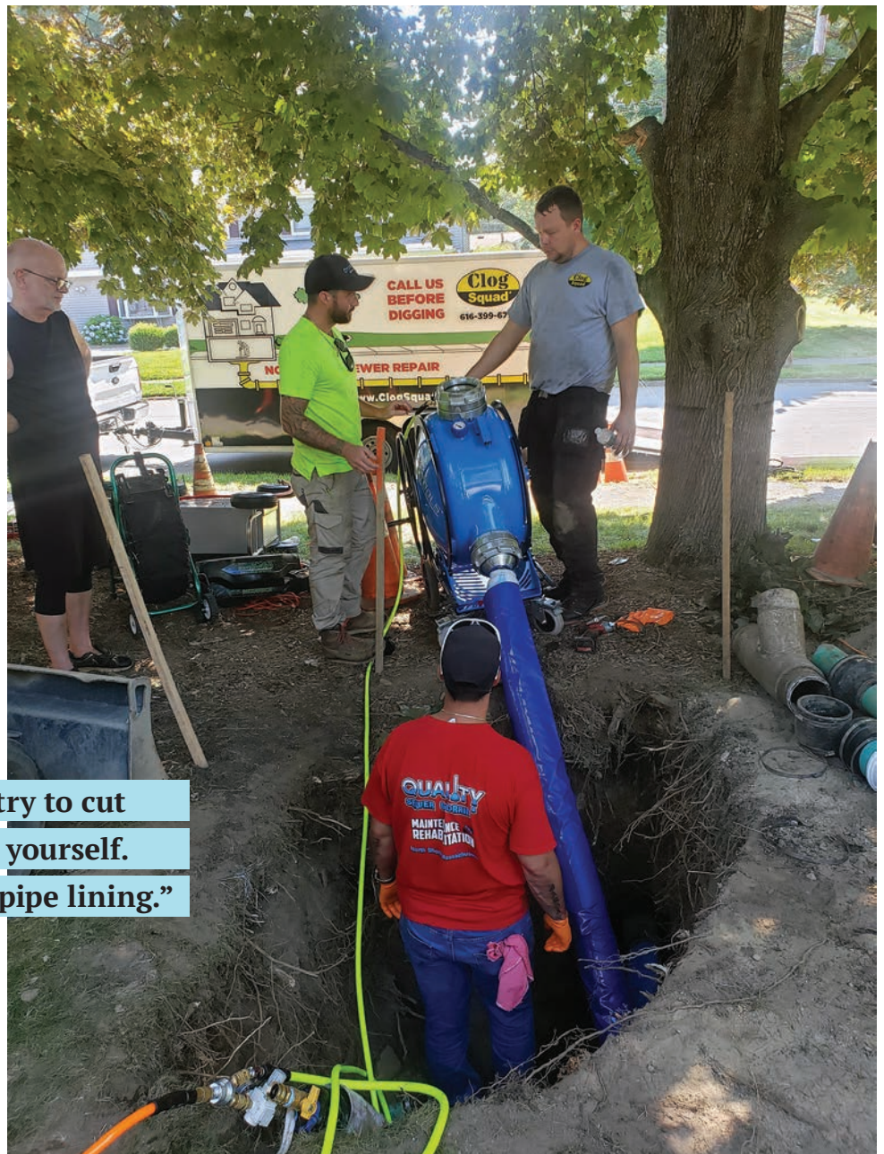
Each one of the four pipe lining projects the crew completed required at least one excavation pit.
