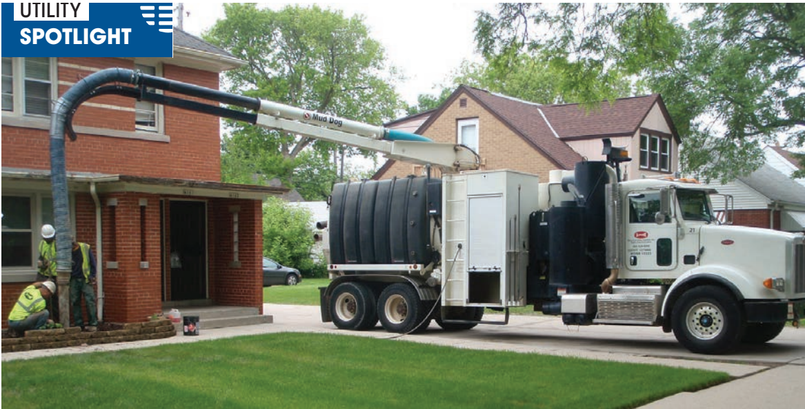
Workers use a Mud Dog vacuum excavator by Super Products during a lateral CIPP repair job in one of Milwaukee Metropolitan Sewerage District's residential areas.
