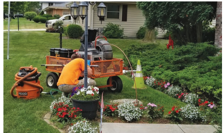
A sewer worker uses a RIDGID SeeSnake to inspect a residential sewer lateral as part of a CIPP repair job.
