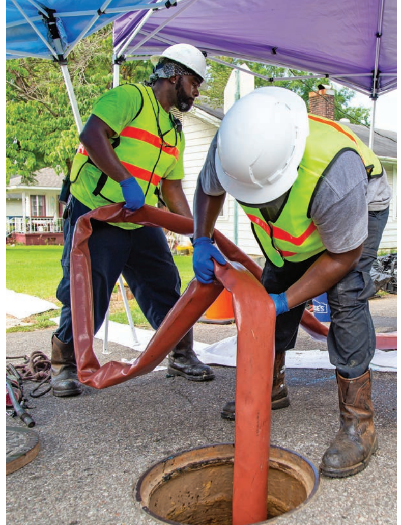
Technicians Anthony Smith (left) and Brandin Burton feed a lateral liner into a manhole.
