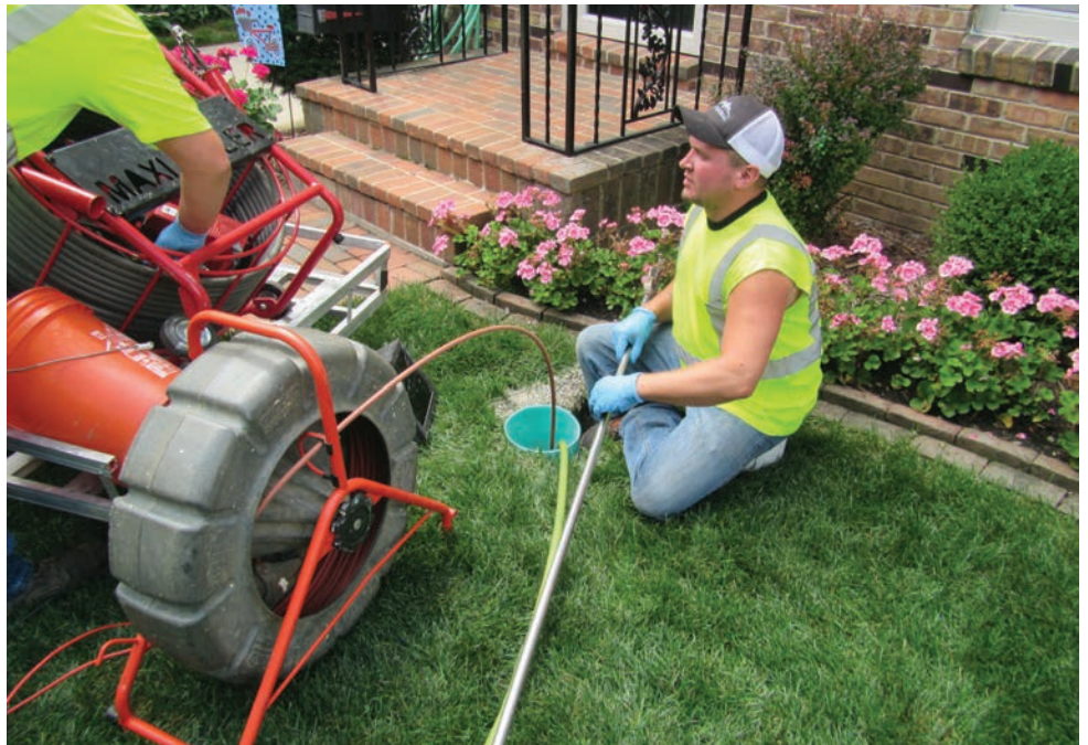
Crews employ a RIDGID SeeSnake as part of a residential lateral pipe repair project in Whitefish Bay.
