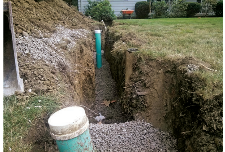
A new conduit financing program provided by Avon Lake Regional Water with the help of the Ohio EPA is allowing customers to address root intrusion and other inflow and infiltration-related issues in their sewer laterals.
