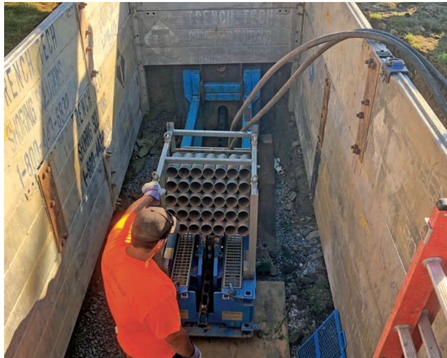
PHOTO COURTESY OF PENN TOWNSHIP SEWAGE AUTHORITY
