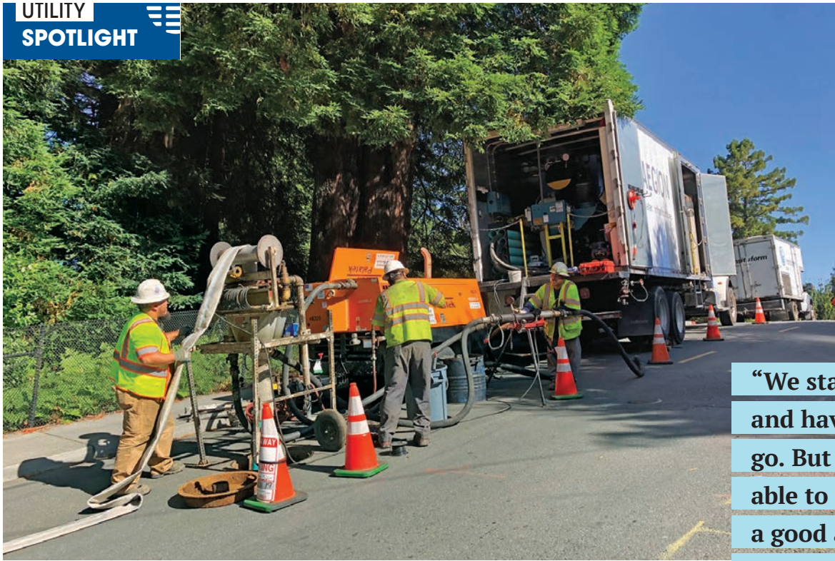
Subcontractor Aegion Insituform installs heat-cured CIPP liners in sewer mains for the city of Arcata, California.
