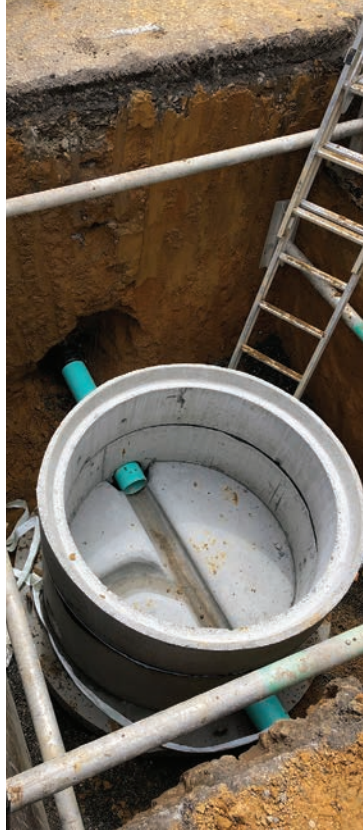
Inflow and infiltration specialist Michels subcontracted on the project to seal 22 leaking manholes by spray-applying SewperCoat PG sealant.
