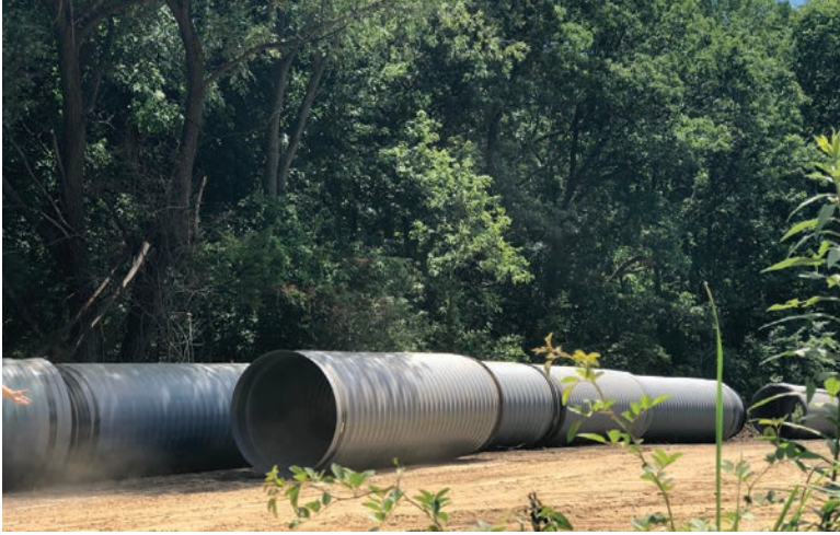
The workers used 48- and 60-inch-diameter SaniTite HP pipe manufactured by Advanced Drainage Systems.
