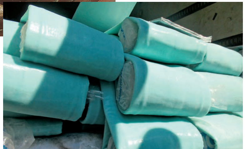
Workers placed the cured-in-place pipe liners on ice to slow the curing process.
