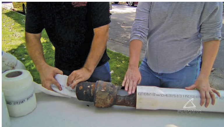
A video on the website shows a plumber inserting a liner into an old steel pipe while a collections system worker looks on and asks questions about the installation.
