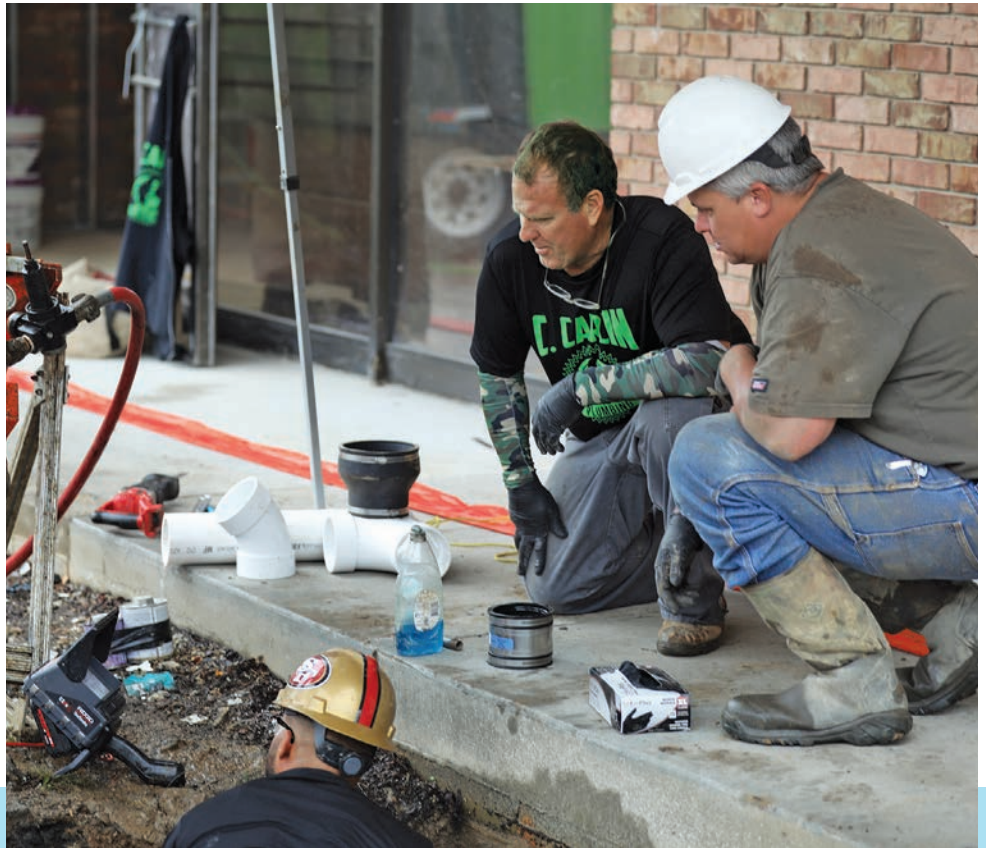
Chris Carlin (center) supervises a large commercial project in which his team rehabilitates a sewer pipe using a CIPP relining system. He believes diversified services are the key to a successful operation and recommends plumbers consider pivoting into more I&I work.
