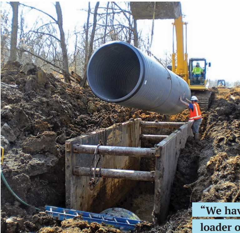
Nearly 2,200 feet of thermoplastic pipe was installed to build an equalization basin to address infiltration and overflow issues in the township of Bath, Michigan.
