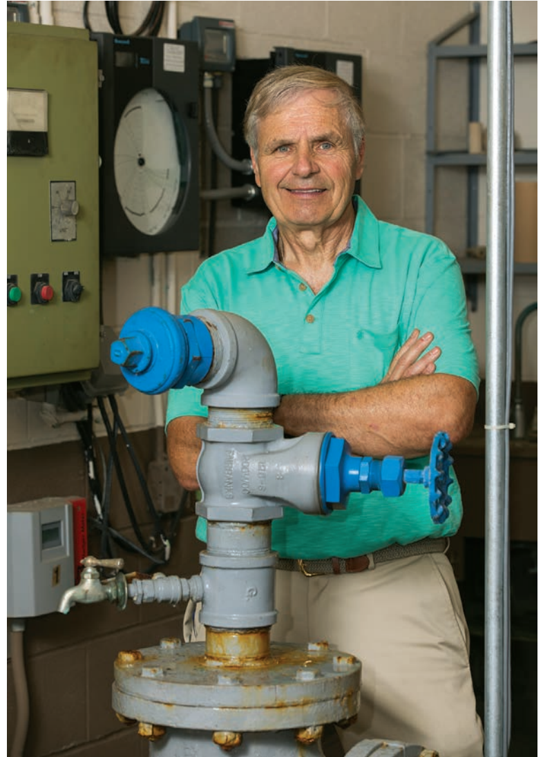
Ray Jarema oversees the operations of the Berlin Water Commission's wastewater collections system.
