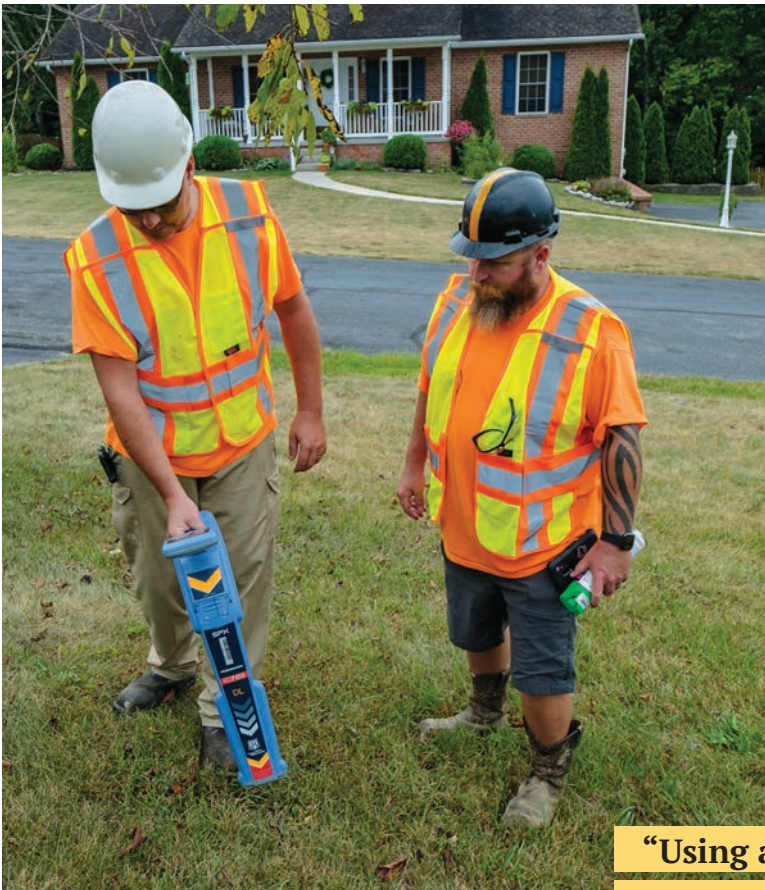
Brandon Dice (left) and Todd Hummer use an RD7100 locator (Radiodetection) to pinpoint the camera's location in a lateral line and mark where they have to dig for repairs.
