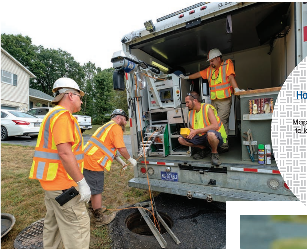
From left, Brandon Dice, Todd Hummer, Justin Hollenshead and Joshua Eyer discuss sewer repair plans while retrieving the inspection camera.
