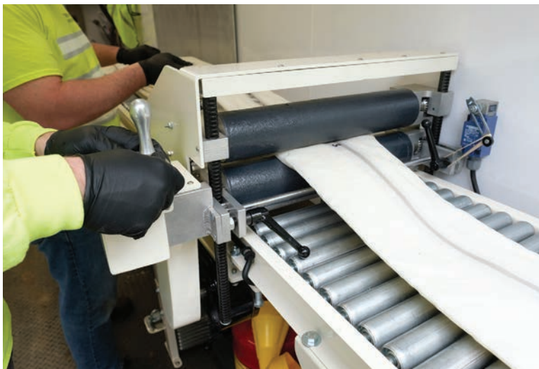
The study sought to determine how long rehabilitation products will remain effective for reducing groundwater infiltration as originally designed.
