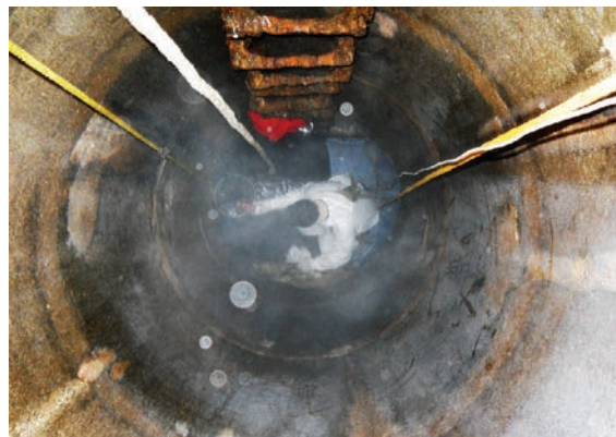
A Naperville Water Department crew member sets up at the bottom of a manhole for rehabilitation work.
