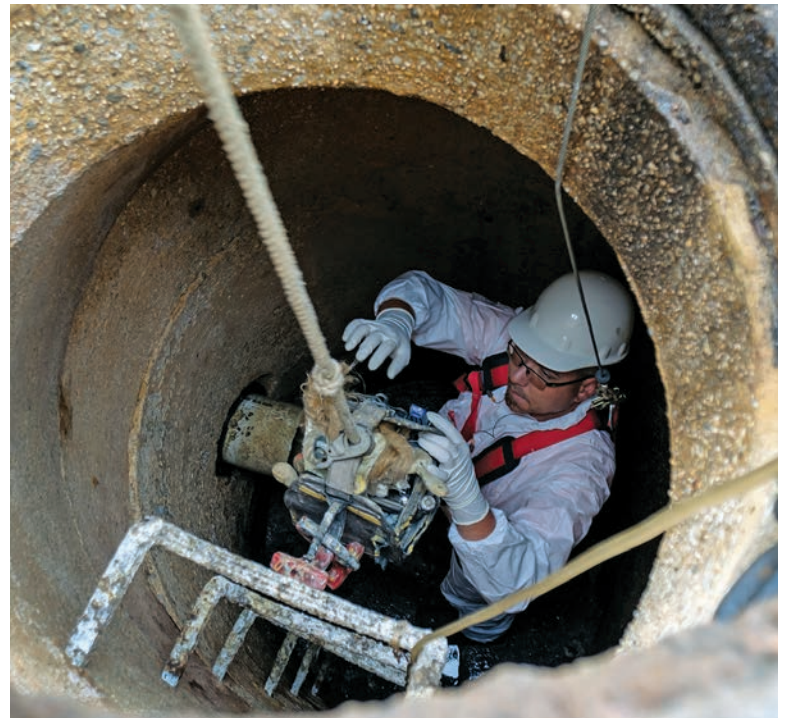
Dice inspects a leaking manhole.
