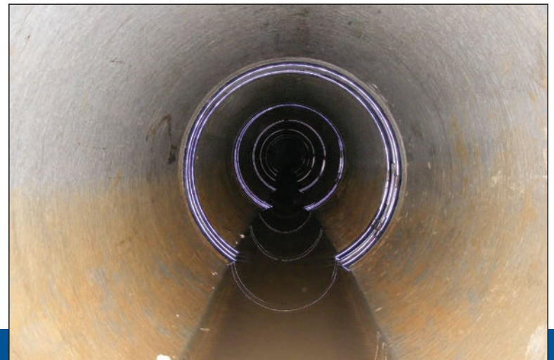
A view down the pipe after 473 HydraTite internal joint seals were installed to eliminate infiltration without full rehabilitation or excavation.
