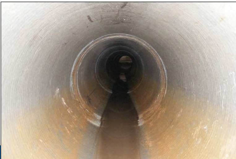
When an Ohio utility discovered a new 36-inch pipe was leaking at all 473 joints before it was even put into service, full rehabilitation and complete replacement seemed like the only options.
