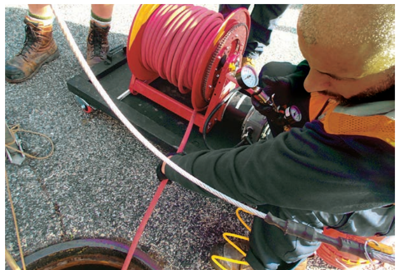
A crew member monitors air pressure to the packer while installing a Quick-Lock repair sleeve.
