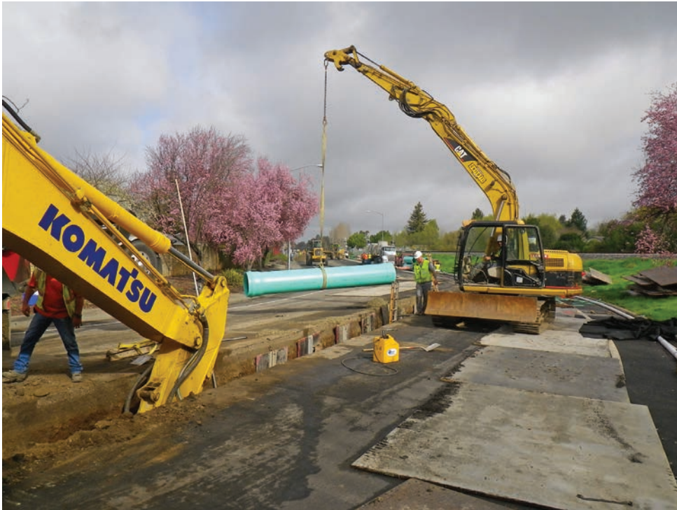
The Rohnert Park sewer expansion project called for open-cut construction, with the use of monolithic base inserts in the manholes.
