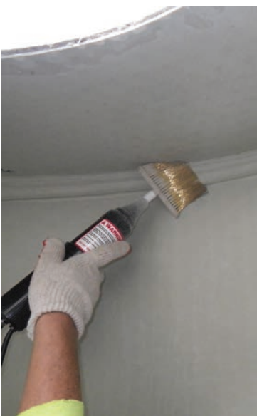
The manholes are designed to have a continuous liner from the base up through the top. Spark testing is used to identify any holes in the liner that require repair.
