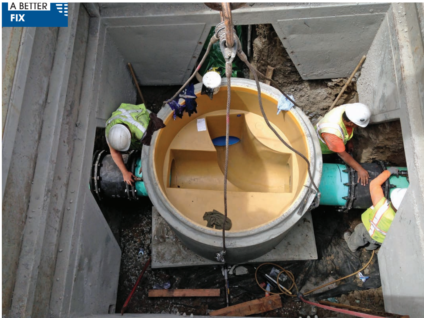
The crew connects a precast base with fiberglass insert and coupled new pipe stubs to an existing sewer main in Rohnert Park, California. The connection to the existing main at left is an intentional overflow connection, with primary flow moving from the right to the top of the photo.
