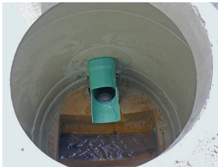
A small-diameter drop connection in the manhole, where the fiberglass base insert was designed to convey flow from the drop to the main channel.
